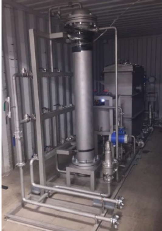
Alberta lithium project; very first 75 bpd pilot plant
